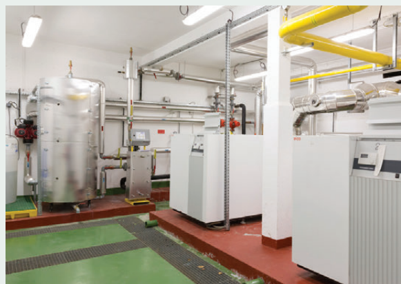
Engie boiler plant at Ris Orangis (91)
