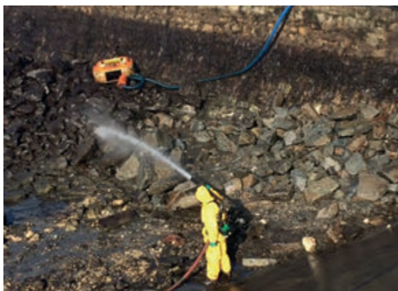
Hosing of riprap following an oil spill. ©Séché
