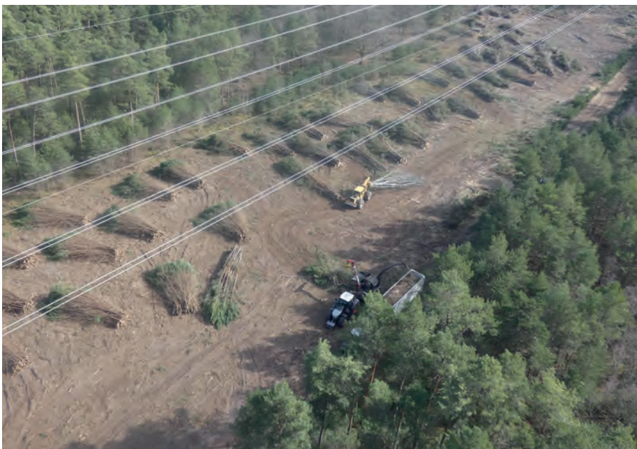
Valorisation of wood cut under RTE cables in the municipality of Nevoy (45).
